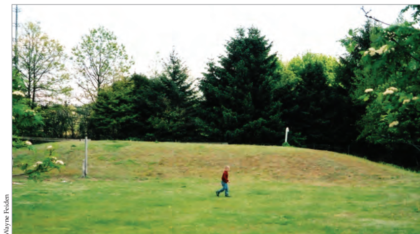
Figure 13. A sand-filled mound system dominating the yard in Hatfield, Massachusetts.
