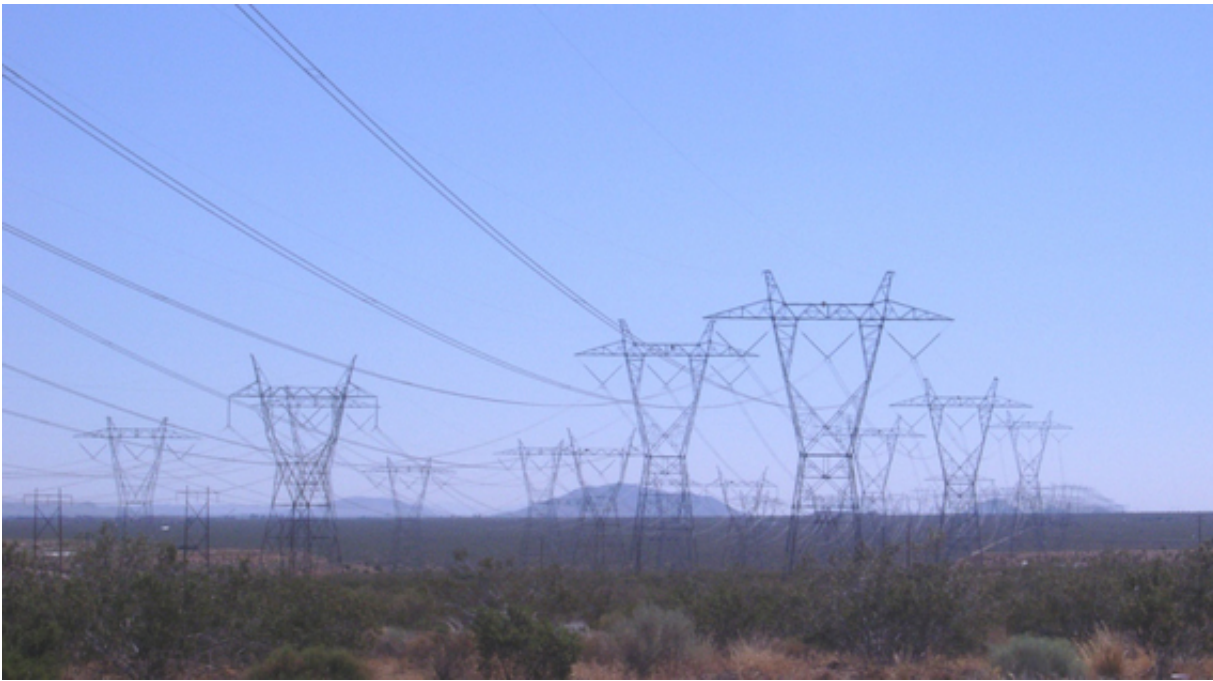
Power generated at central-station facilities must be transmitted over high-voltage power lines such as these, which run through California's Antelope Valley. Photo by Josh Hohn.
