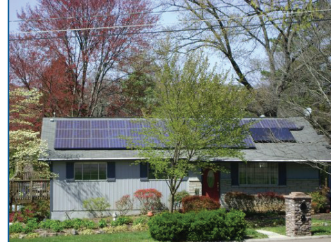
A PV System installed on a residence. (Photo credit: Courtesy of DOE/NREL)
