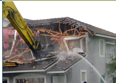
A Florida court ordered the demolition of these multifamily buildings because they were inconsistent with the comprehensive plan. (Image credit: Jim Nicholas)
