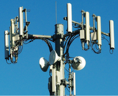
Multiple antennas on a single monopole tower on Sexton Mountain in Beaverton, Oregon.
