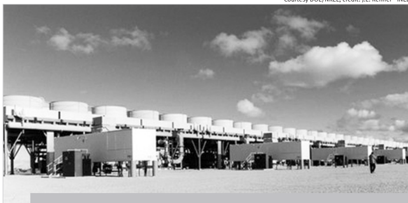
☺ The Soda Lake Power Plant 2 in Soda Lake, Nevada, has a 12 MW capacity.
