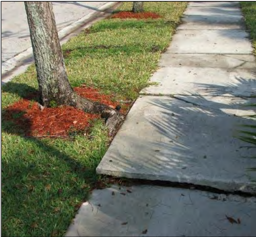
Broken and lifted sidewalks
