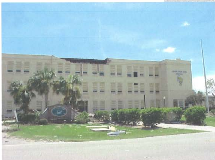
CHARLOTTE HIGH SCHOOL'S HISTORIC BUILDING WAS HEAVILY DAMAGED AND UNUSABLE FOR A LEAST A YEAR.
