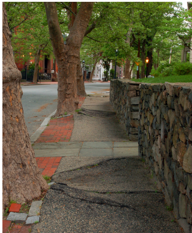
Figure 2.4. Uneven and broken sidewalks pose barriers to accessibility (Kirkikis/Getty Images)
