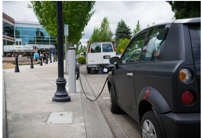
Figure 2.7. On-street EV charging station in Hillsboro, Oregon (Visitor7/Wikimedia Commons CC BY-SA 3.0)
