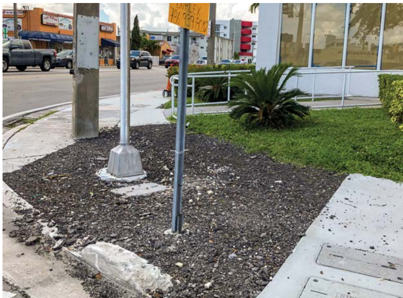
Create temporary curb ramps during construction projects (something that was not done in the above photo) to avoid limiting mobility options.
