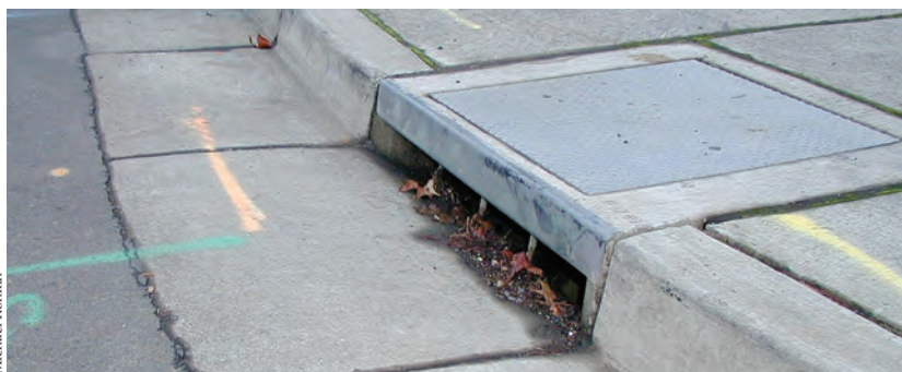
Figure 7.33. A drainage grate
